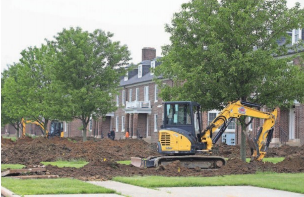
East Gate will soon be a neighborhood of 68 restored officers' homes at Fort Monmouth in Oceanport. PHOTOS BY TANYA BREEN/STAFF PHOTOGRAPHER
